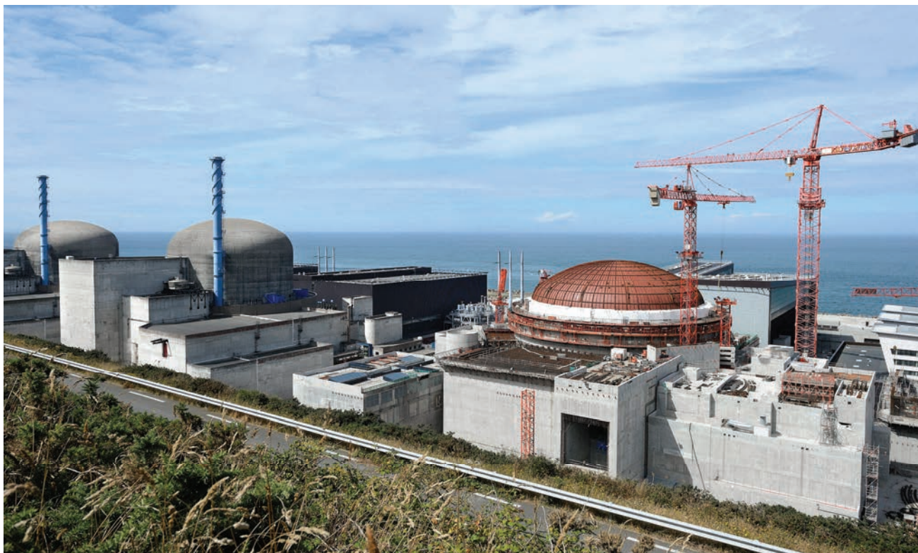
Flamanville site—EPR construction (unit 3) and 2 1300MW operating units, France, August 2013 (EDF, Alexis Morin).
