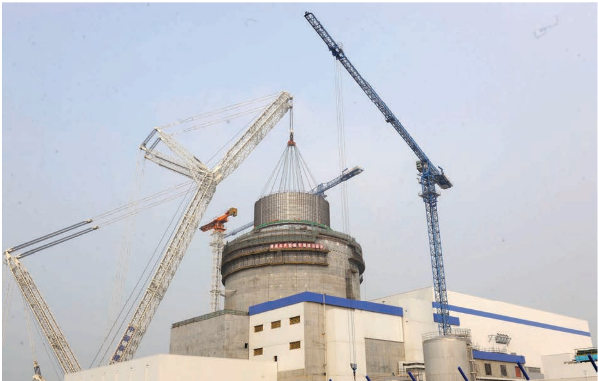
Haiyang Unit 1—Installation of CB20 module, AP 1000, People's Republic of China, March 2014.
