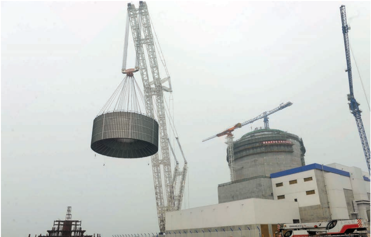
Haiyang Unit 1—Installation of CB20 module, AP 1000, People's Republic of China, March 2014.
