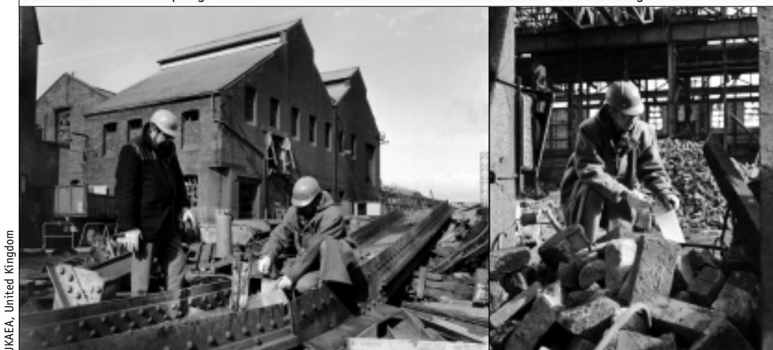
The radiation protection system has evolved over the years. The photos here show workers in the 1970s checking for release of toxic material during cutting-up operations on steelwork, and sampling firebrick from a demolished furnace at Harwell in the United Kingdom.
